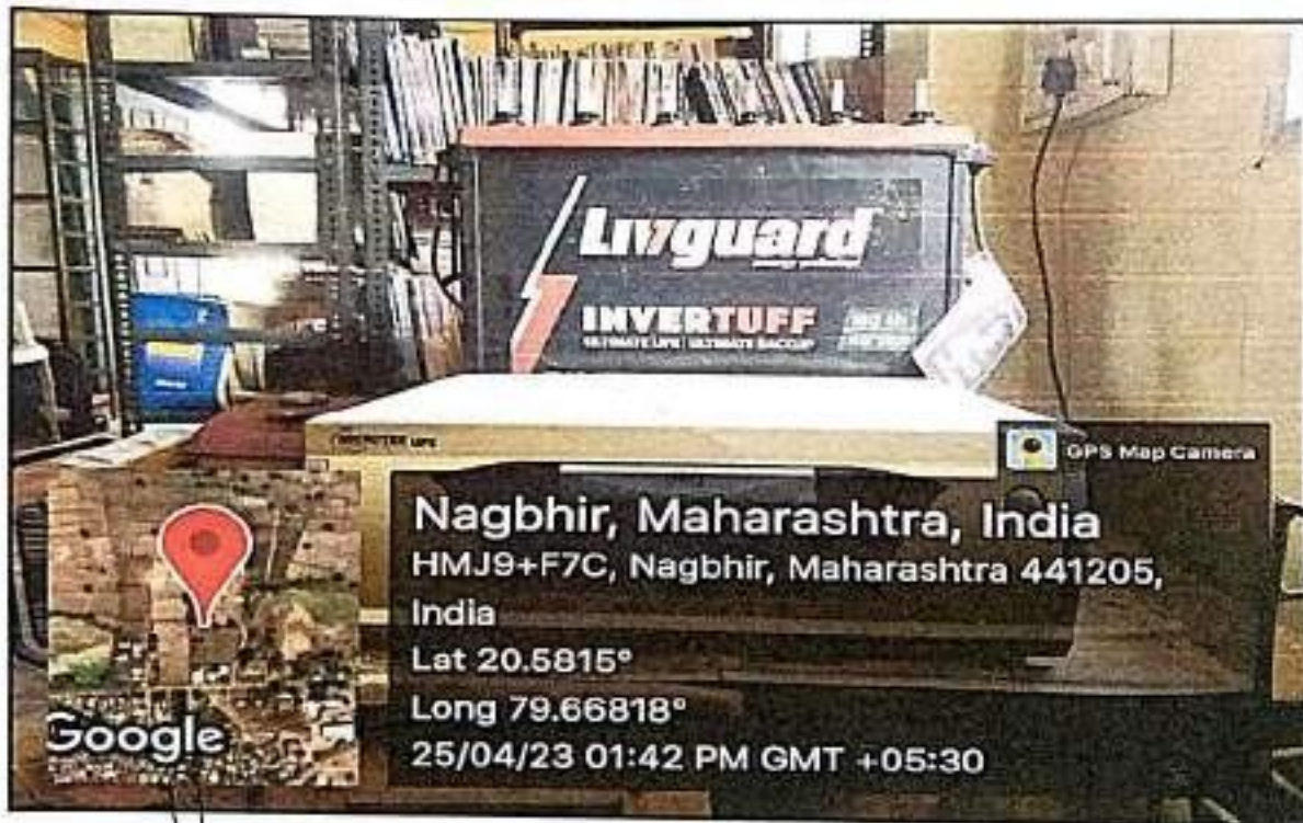
7.1.2 ENERGY STORAGE INVERTER
