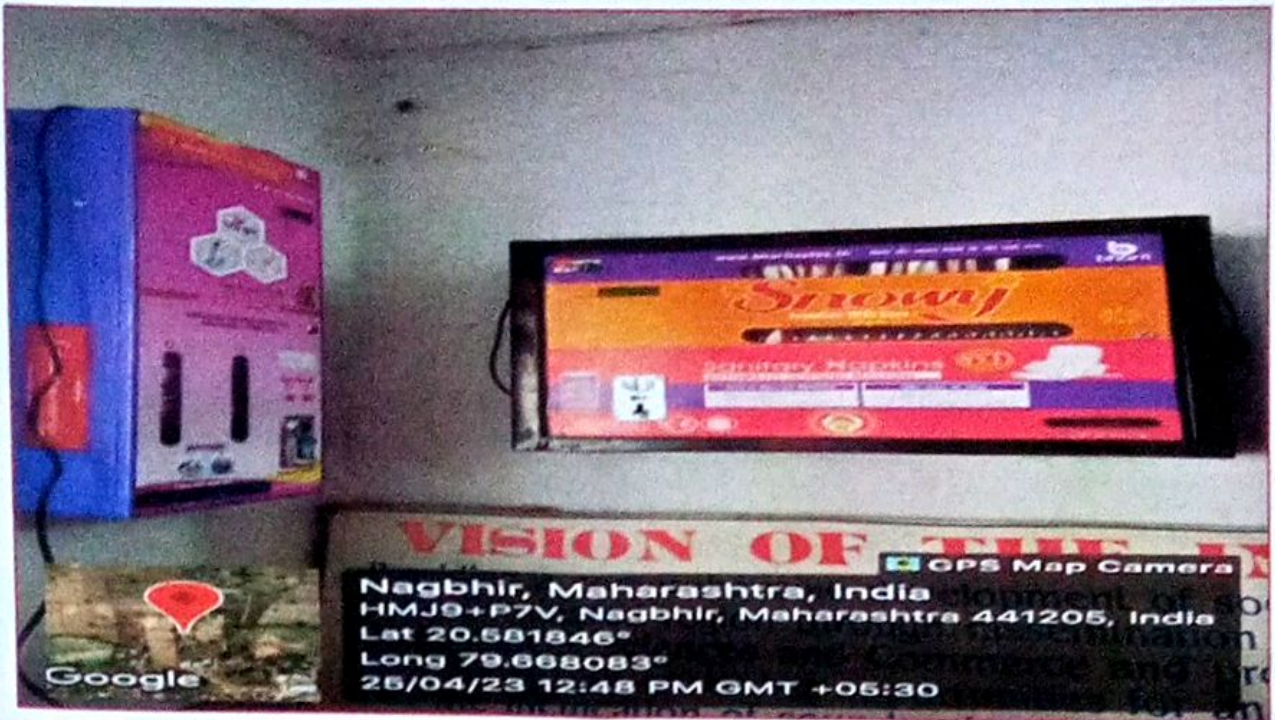
Automatic Vending Machine Installation in the Girls Common Room
